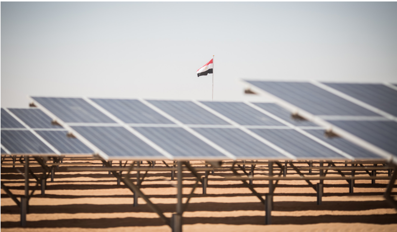
Photo above: The Egyptian flag flies over solar panels during the inauguration ceremony for the first stage of the Infinity 50 Solar Park near Aswan, southern Egypt, on March 13, 2018. Photo by Oliver Weiken/picture alliance via Getty Images.
