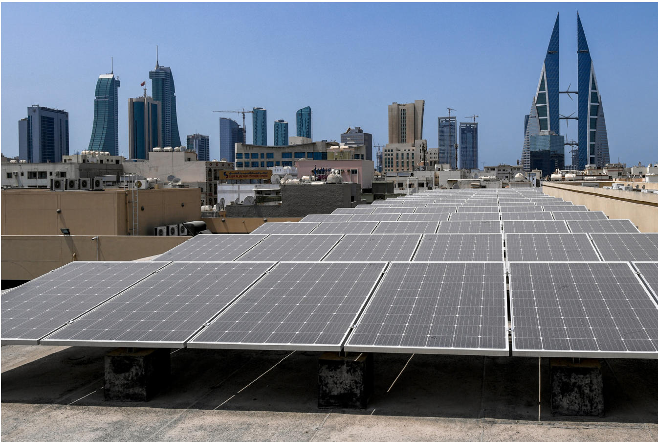
Photo above: Solar panels are installed on the roof of a school in Bahrain’s capital Manama on Aug. 25, 2022. Photo by MAZEN MAHDI/AFP via Getty Images.
