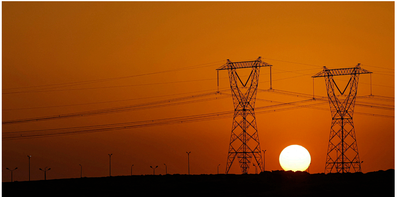
Photo above: High-voltage transmission towers run along a highway in El-Shorouk, Egypt. Photo by KHALED DESOUKI/AFP via Getty Images.
