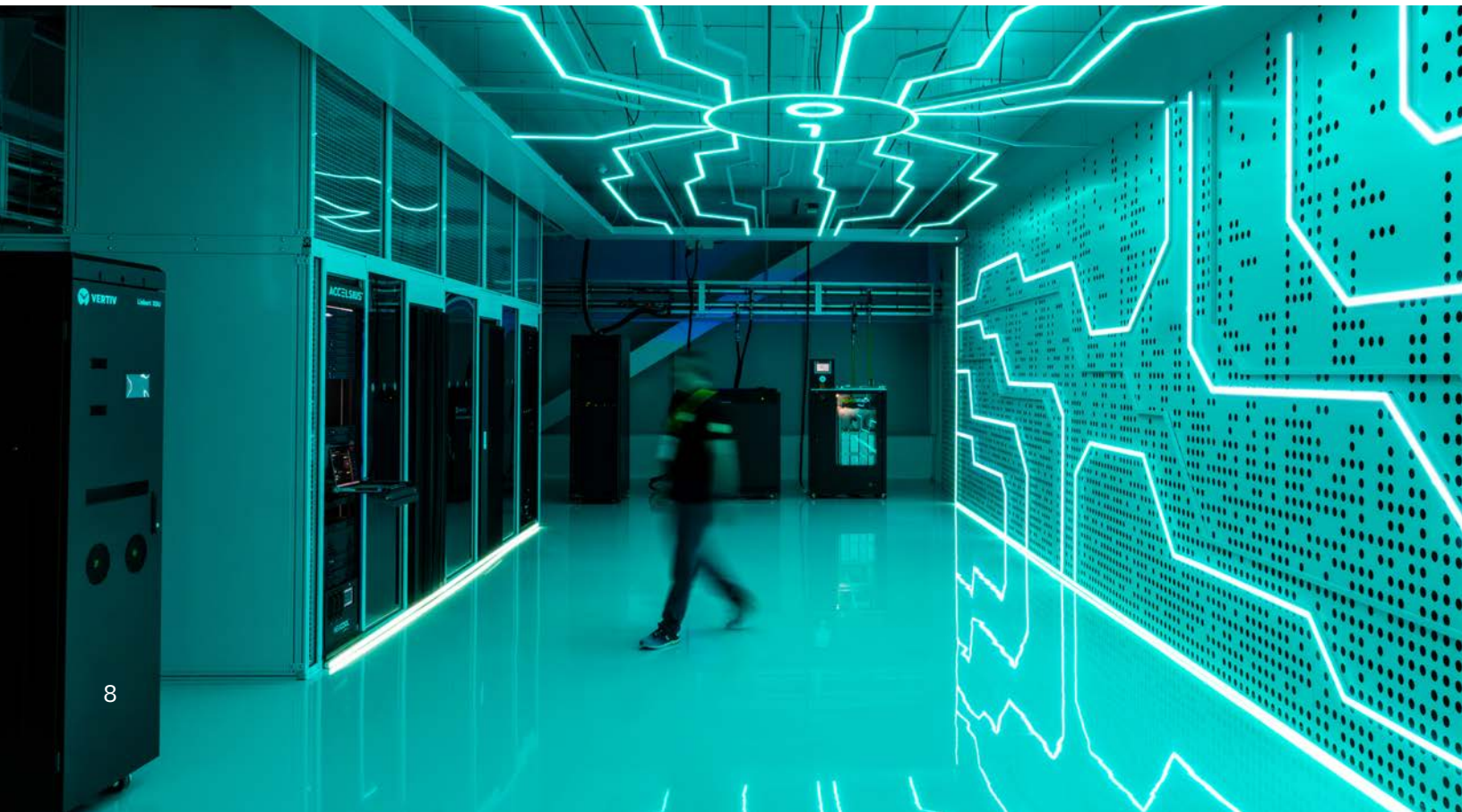
Liquid cooled servers in an installation at the Global Switch Docklands data center campus in London, United Kingdom, on June 16, 2025. Photo by Jason Alden/Bloomberg via Getty Images.
