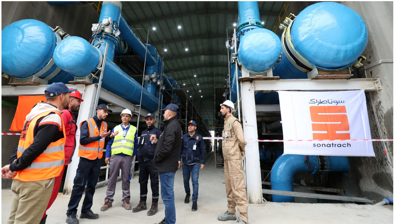
Photo above: A seawater desalination plant in Oran, Algeria, on February 20, 2025. Source: Billel Bensalem/APP via Getty Images.
