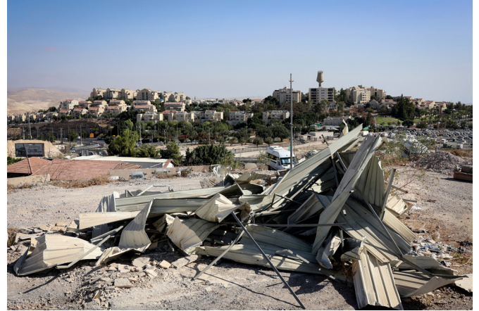
Demolished Palestinian home in the West Bank with the Israeli settlement of Maale Adumim in the background, on September 30, 2025. Source: Zain Jaafar/AFP via Getty Images.
